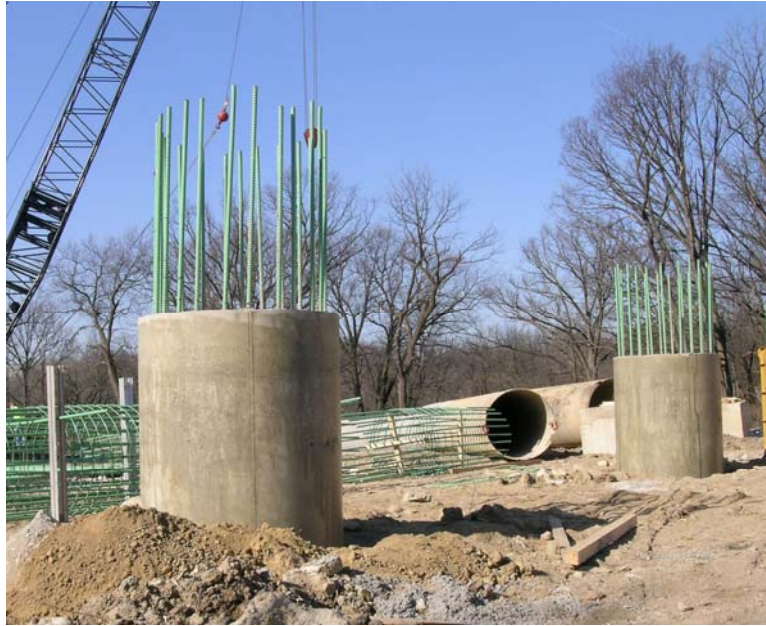
These pier footings are ready for the next concrete pour. Each pier consists of four support columns, topped with a pier cap.
